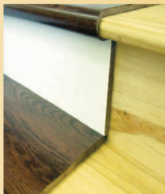
The StareCasing solid hardwood treads and risers fit neatly over the existing stairs — careful measurement is key to a perfect installation.
